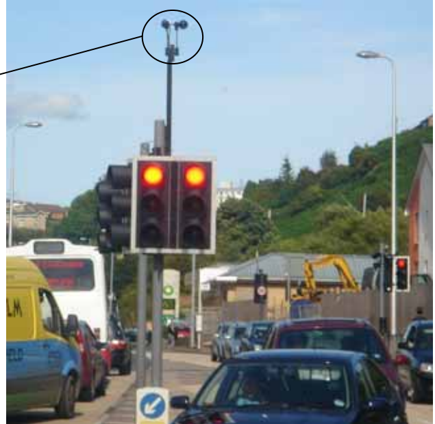
A TrafiCam installation in Greenock, UK.
